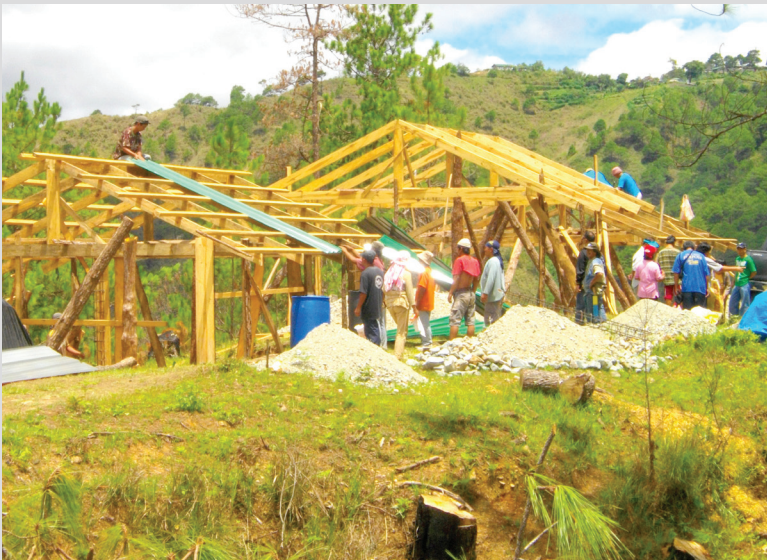
"Gamal" (cooperative endeavor) in Labey, Benguet, to build houses for families affected by the landslides in 2009
