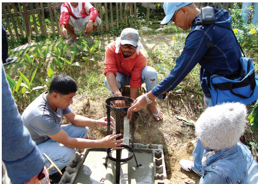
Installation of rain-gauge in Maragusan. ACCORD helped partner municipalities establish community-based early warning systems.
