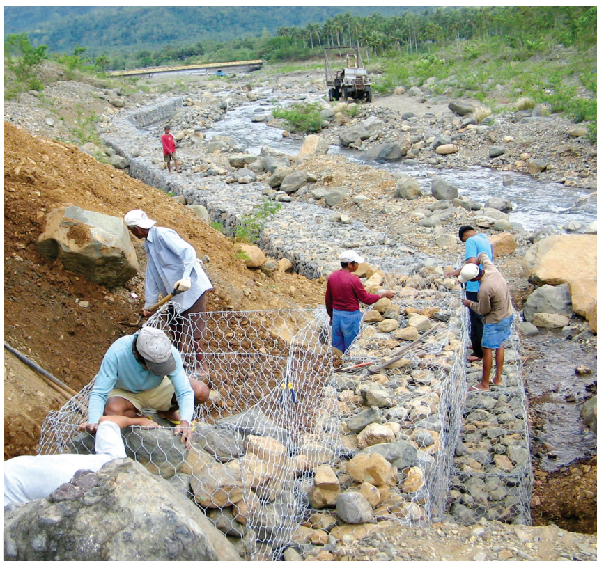
"Bayanihan" of residents of Bgy. Davil-davilan in Dingalan to fill the Gabion boxes with stones which will serve as flood mitigation.
